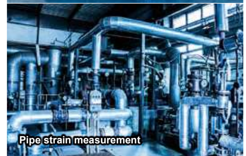
Brake and pipe strain measurement
